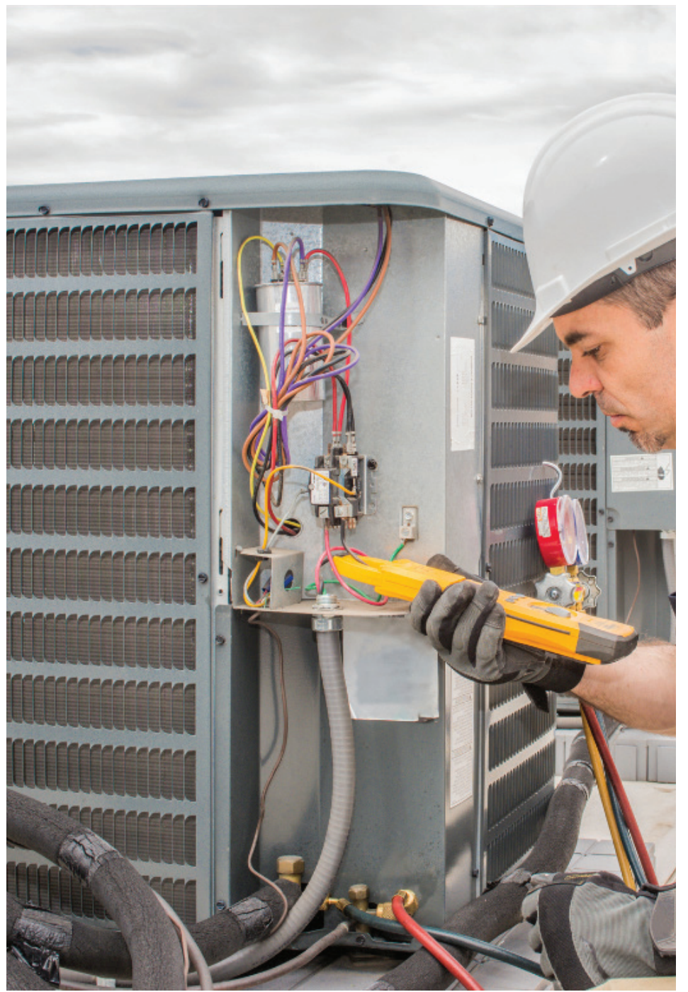
Ensure your air conditioning system is ready for the approaching summer by asking your HVAC professional about Cotton Electric's Spring Tune-Up Rebate program.
